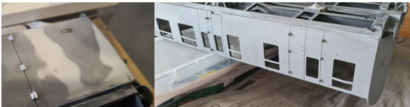
A final flaw filled and, on the right, another coach ready for the top coat.
