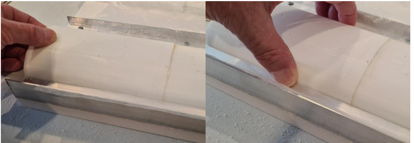
Fitting the panels into the jig ensuring that they are hard up against their neighbour as they are slotted in to prevent the polythene riding up into the joint. Compressing the panel on the right allows it to clip into place between the angles. These then hold and align the panels firmly.
