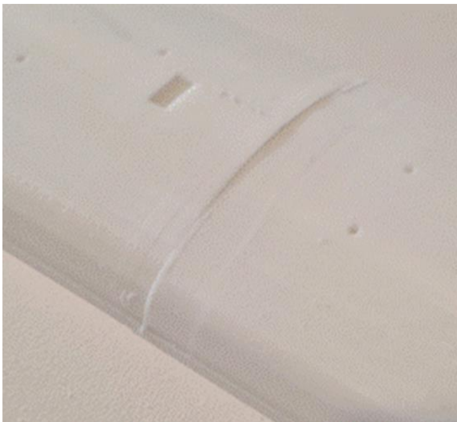
The slight misalignment in the joints and somewhat rough finish is apparent
