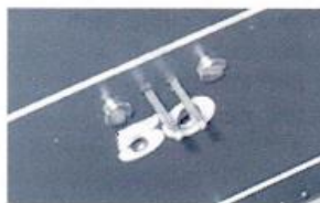
Figure 6: External power plug at the back of the engine
