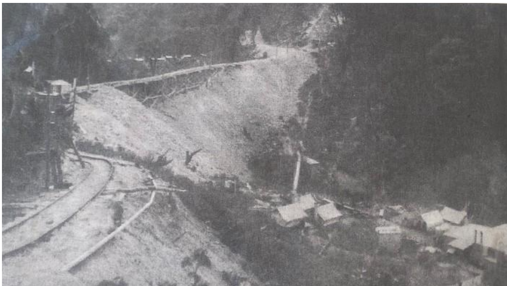
Construction photos of the large timber trestle viaducts, you would not realize that you were passing over these as their very existence is now hidden with earth. Apparently the timber has been tested and still structurally sound.
